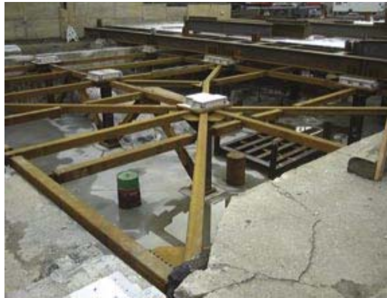
Steel transfer girders at the first floor level are supported by isolators made of springs, rubber, and Teflon.
