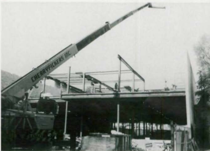
By using composite construction with partially restrained connections, the project's designer reduced the typical girder size from W14x34 to W14x22. The RGS design also reduced the number of studs required, though it did require the member to be cambered.
